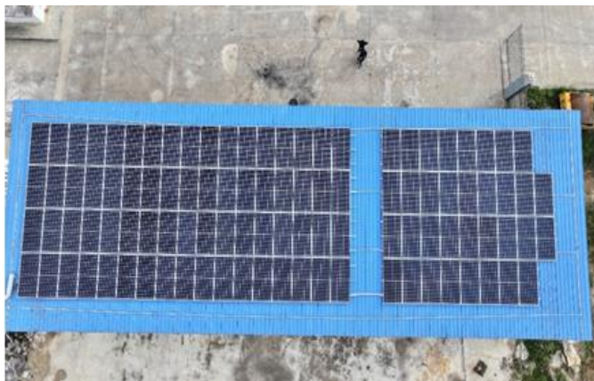
Figure 3: Solar Panel Installed
